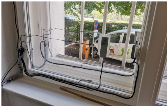
Figure 6: top: one of the examined case-study buildings; bottom: Monitoring equipment in a vacuum-glass equipped casement window (source: the authors)
